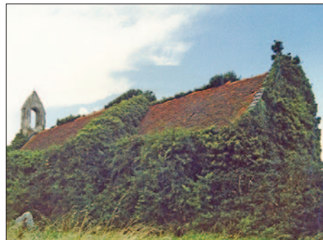
▼ St Denis' in 2002: covered in ivy and in danger of collapse.
