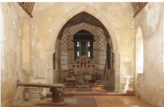
St Denis' church, East Hatley – looking into the chancel. By April next year the walls in the chancel will have been repaired and new windows installed on the north and south sides.
