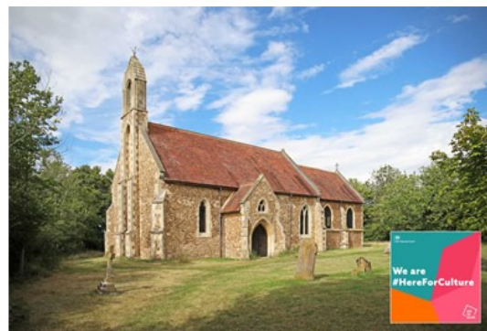
St. Denis' church, East Hatley. Built around 1215 it now belongs to the Friends of Friendless Churches. A grant from #HereForCulture will enable the chancel to be repaired.
